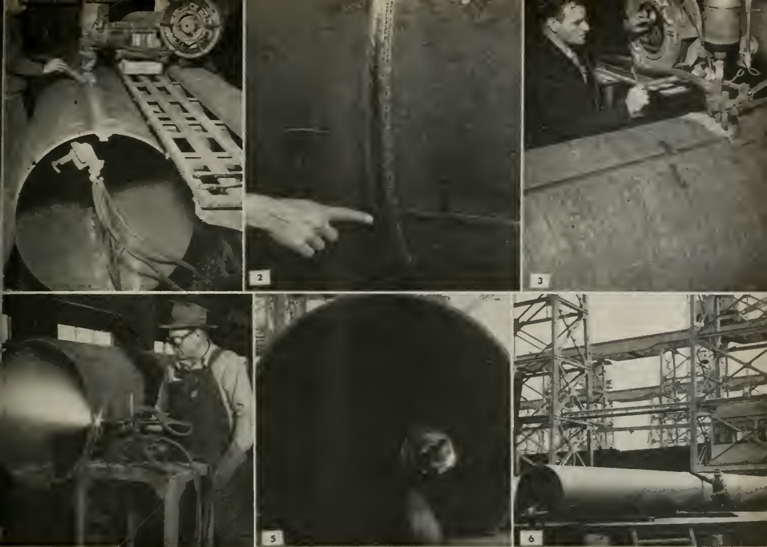
Fig. 1. A longitudinal seam being welded mechanically on two halves of one section. Backing strips, tack-welded on the inside, hold the two halves together while this operation is being performed. Fig. 2. Closeup view showing where longitudinal and circumferential welded seams of two sections meet. Note the unusually clean appearance of the seam. Fig. 3. Two sections of kingposts are shown being welded together circumferentially. Fig. 4. Before kingpost sections are welded together, their ends are burned off square with a 15° bevel, as shown above. Fig. 5. This striking photo, looking into the 61 ft. long kingpost, shows a welder at work welding the backing strip under a circumferential weld where two sections come together. Fig. 6. A completed kingpost. This one is 61 feet 13/8 inches long and weighs approximately 13 tons.
